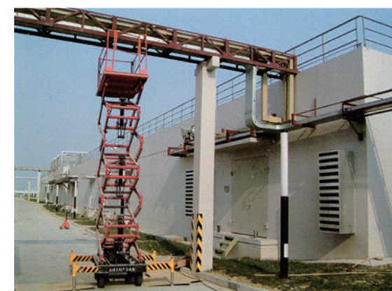
穿墙及并线 Through walls and parallel wires
