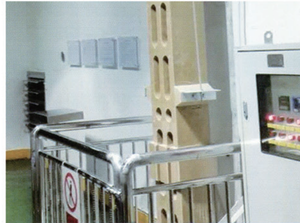
JDR在廊道内的应用 Application in the gallery
